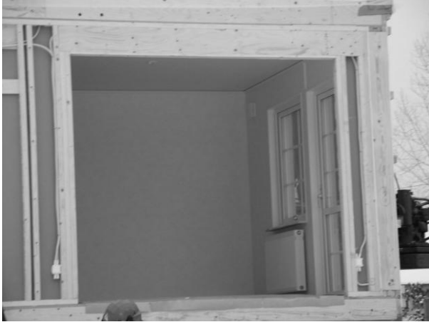
Picture 1: Prefabricated module for single family house with already installed heating and ventilation system and other interior fittings. Arrival on-site.
